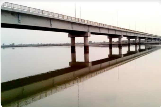
A side view of Structure work of Bridge over River Jhelum at Langawala Pattan District Sargodha.
