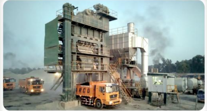
Asphalt Plant Nikko (120 Ton/Hr) Working at N-5, Khanewal.
