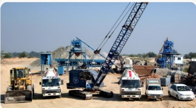
Concrete Batching Plant with Allied Bridge Construction Machinery
