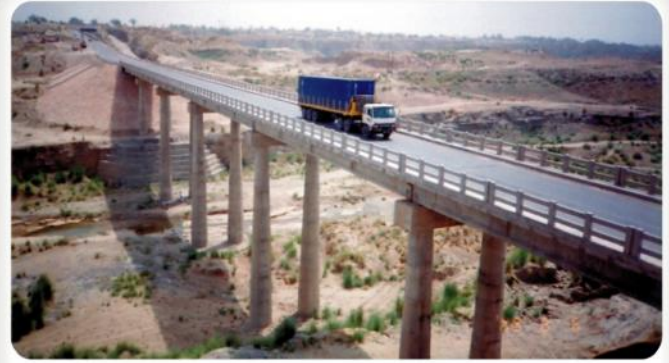
High Level Bridge at Ankar Nullah at Talagang Mianwali Road (Column Height 95 ft)
