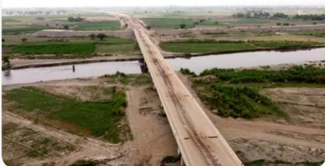
A View of Structure & Approach Road of Mal Fatyana Bridge, Dist. T.T.Singh
